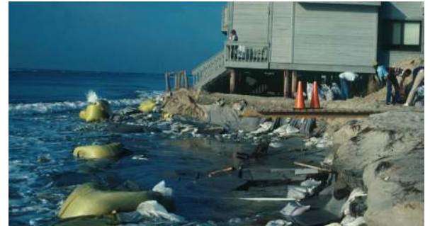
FIGURE 24. Failed, low-cost shore protection. Once punctured, large sand bags leak their contents and are no longer effective.
