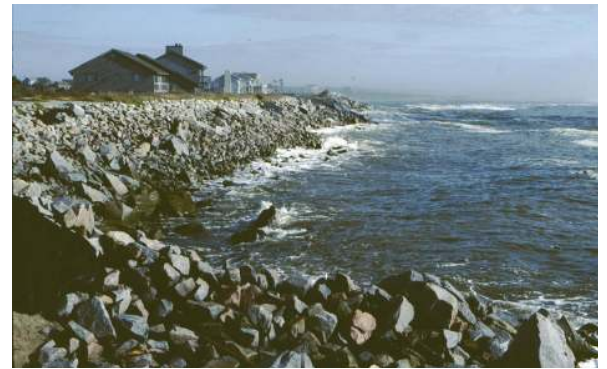
Massive quarry-stone seawall protecting private property (1985) before restoration of the beach – Seabrook Island (SC) [see cover photos]
