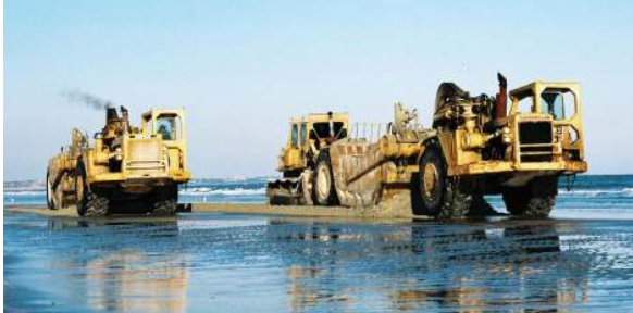
Pan earth movers excavating low-tide terrace in accretion zone for transfer to erosion zone
