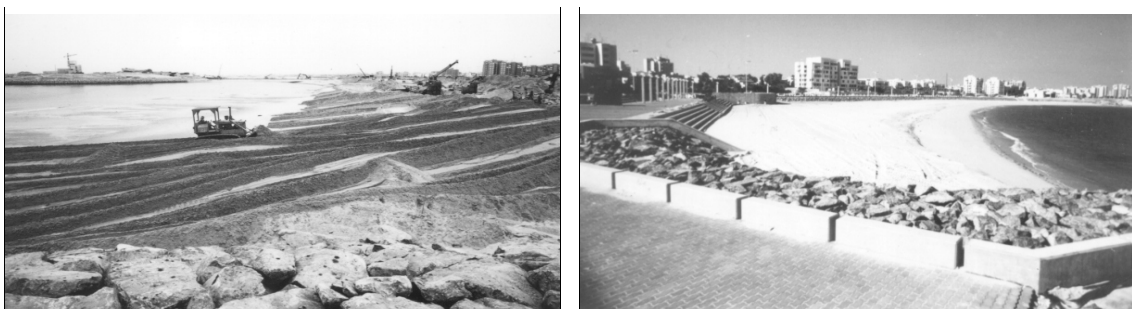
FIGURE 2. Oriented beaches were designed to be retained by “groins,” outfalls that doubled as promenades. Beach-quality sand was imported from inland sites and spread to the design shape.
